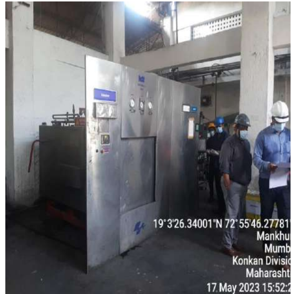
Photograph-10: A view of autoclave for treatment of red category of BMW.
